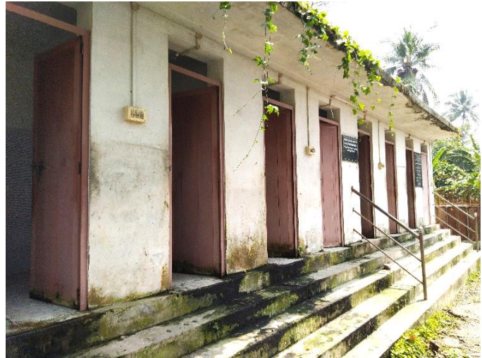
Figure 6.9 Community Toilet Block at Municipal Colony
