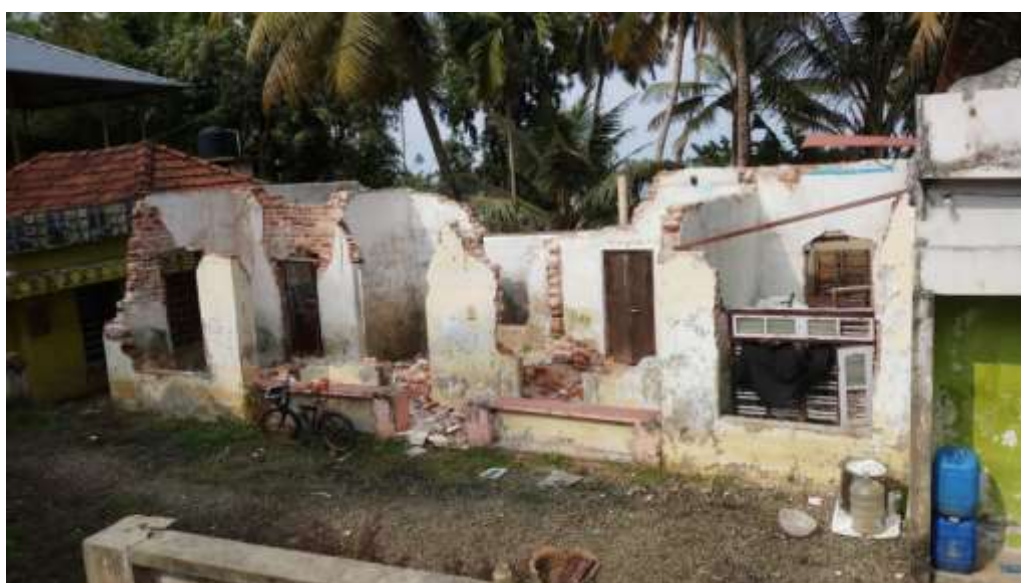
Figure 39: House completely damaged by floods, Primary Survey 2019
